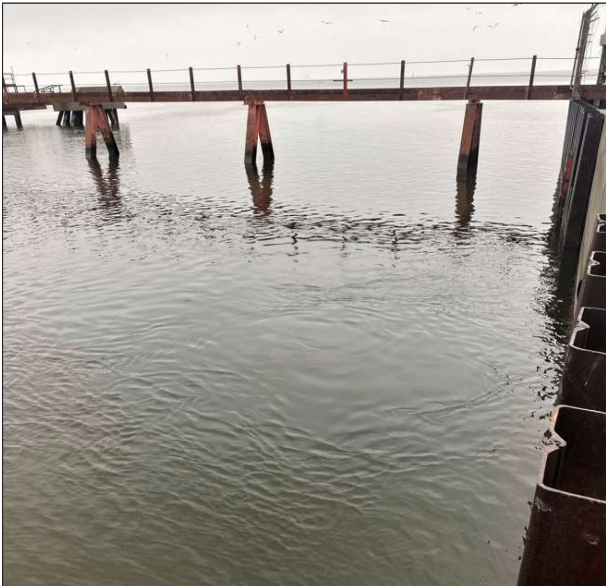
Figure 3-2. Visible Swirling/Roiling in the Fox River above the GBF Outfall (Shorewall is Concrete Structure at Right).
