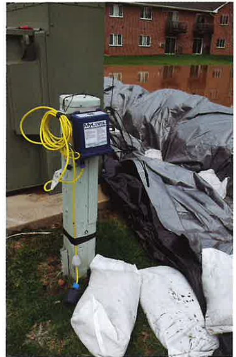
The berm around the ERLS, protecting the transformer, which is the green colored structure in the back. The level monitoring is in the foreground, which indicates if the water level would exceed the berm.
