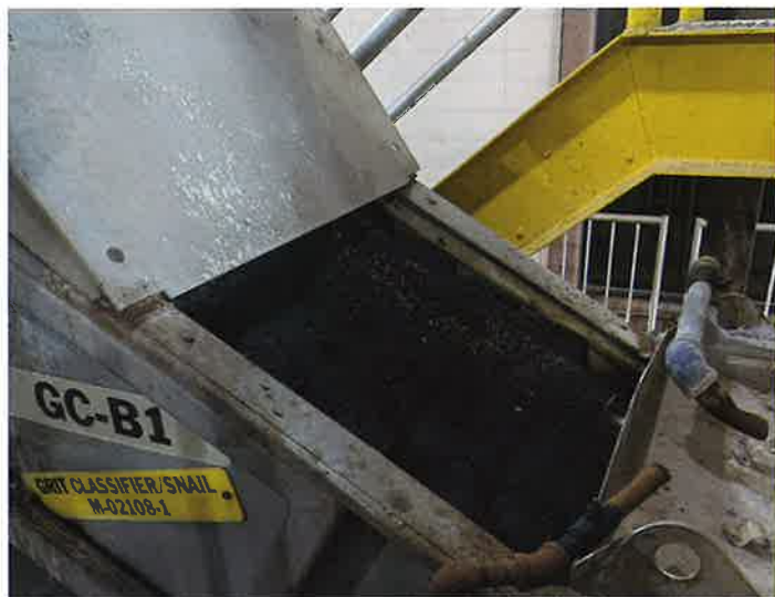
NEW Water's grit classifiers overwhelmed as the surge of grit and chunks of asphalt poured into the plant.
