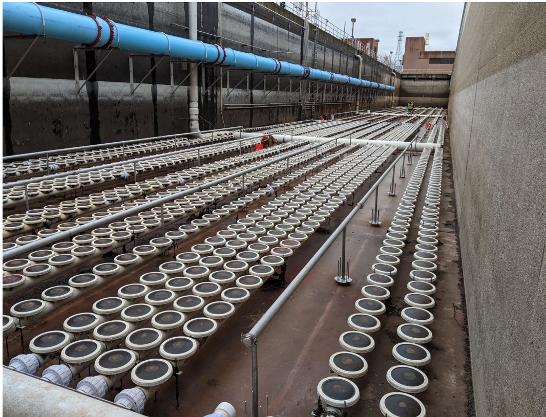
Compressed Gas Mixing Installed in Aeration Zones
