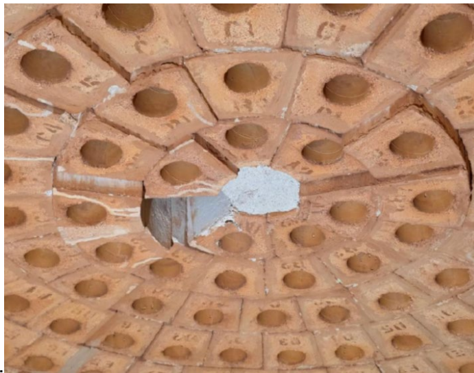
Figure 1 Damaged FBI Refractory Piece
