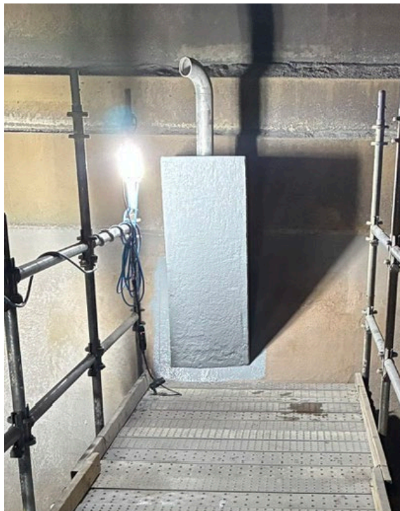
Photo 2 – High-strength waste piping and concrete pad inside of #1 Digester
