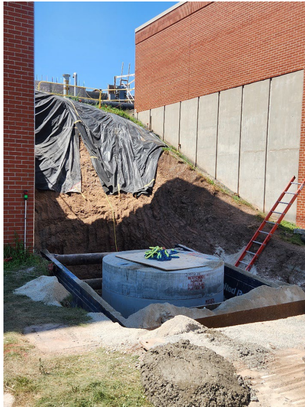
PROCESS RETURN PUMPING STATION
