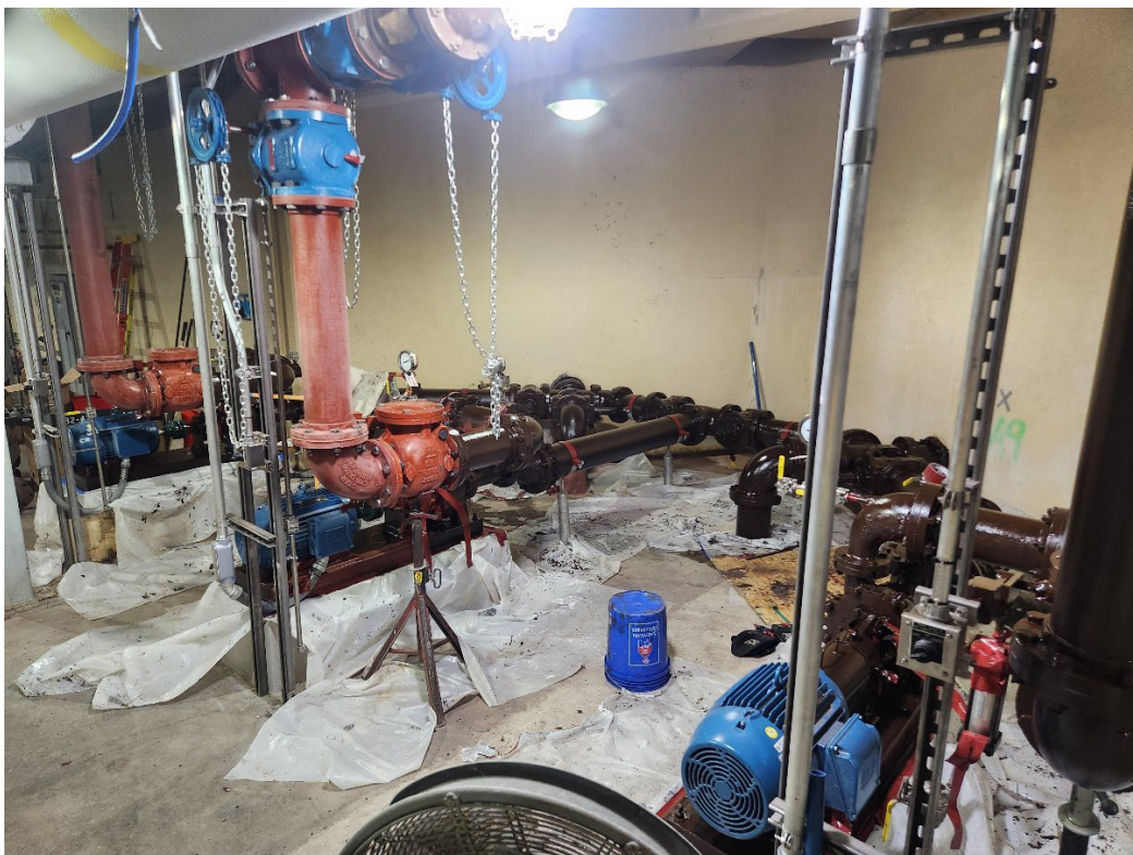
NORTH BANK OF NEW PRIMARY SLUDGE/GRIT PUMPS
