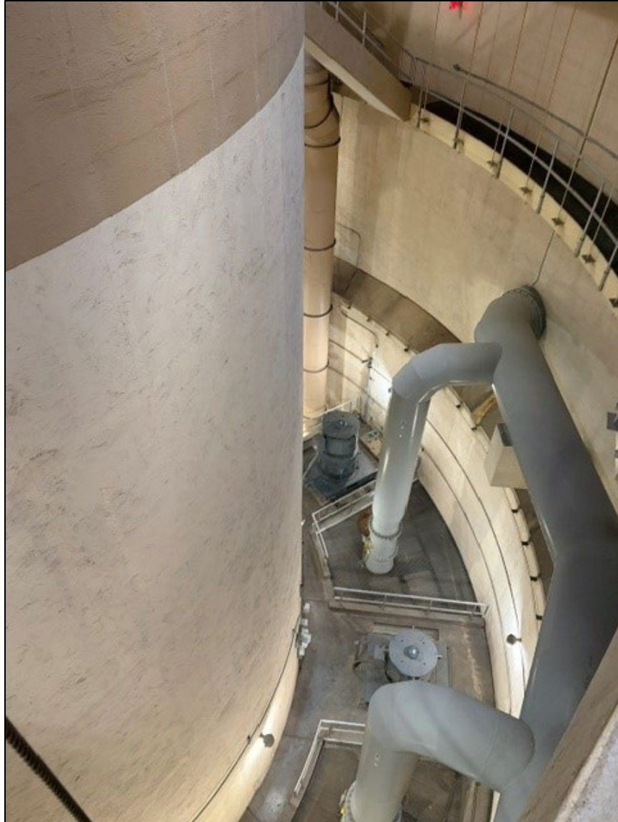
GBF Pump Station
