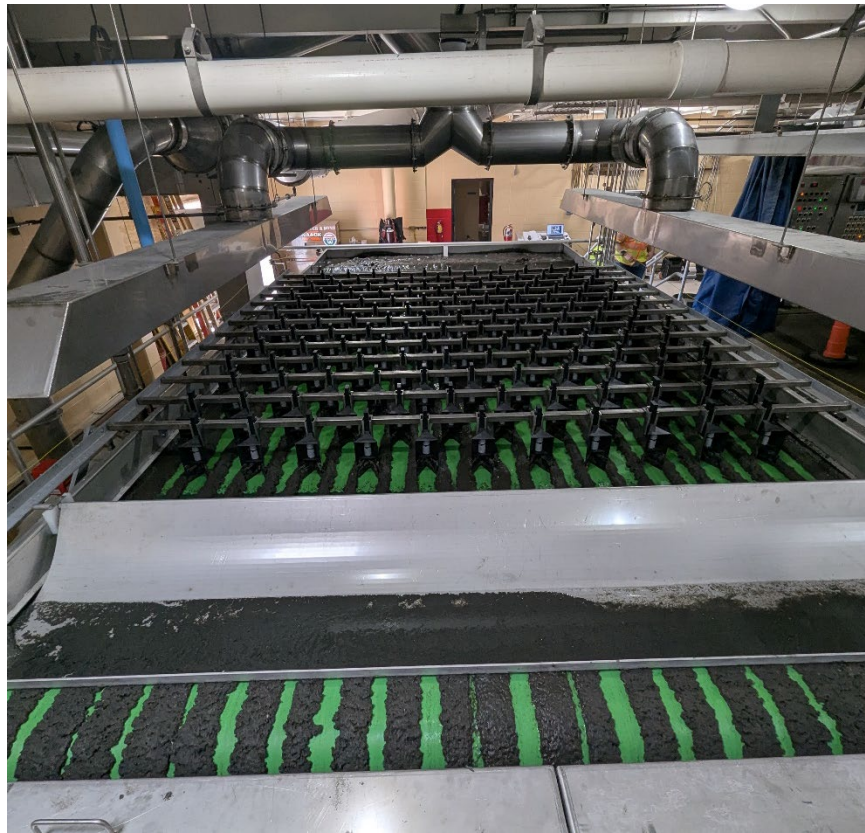
Figure 1: Testing of Gravity Belt Thickener #4
