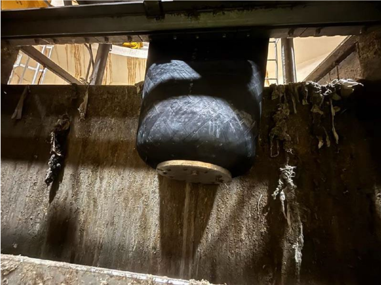
Photo 1 – Sewer Plug being recovered at the top of the bar screen rakes.
