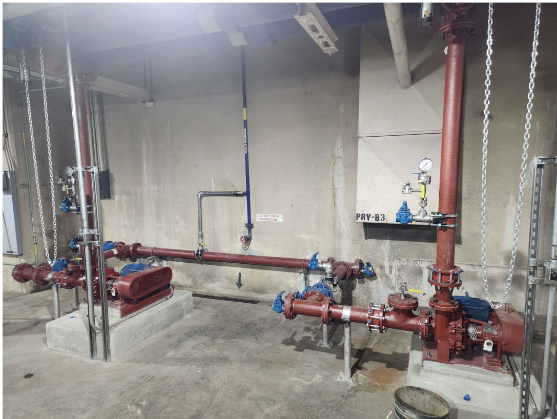
NEW SCUM PUMPS AND PIPING FOR FC #3
