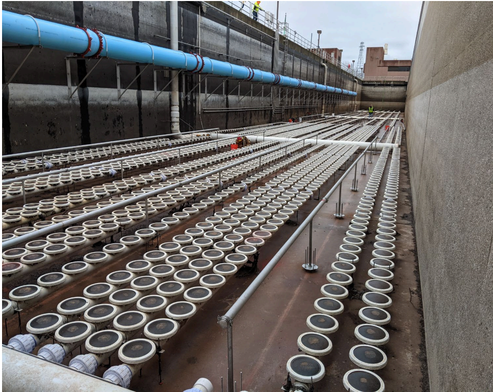
Compressed Gas Mixing Installed in Aeration Zones
