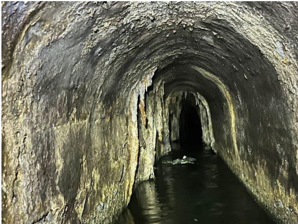
Photo 2 – Calcium buildup in EFR interceptor prior to contractor cleaning efforts.
